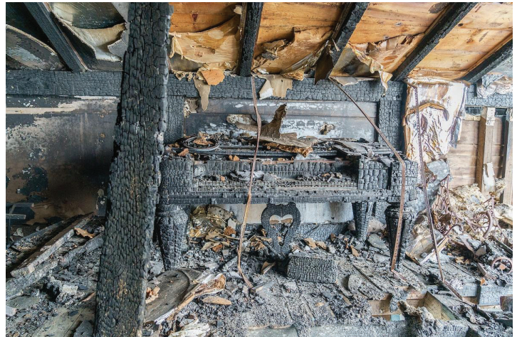
A charred antique piano on the second floor.
