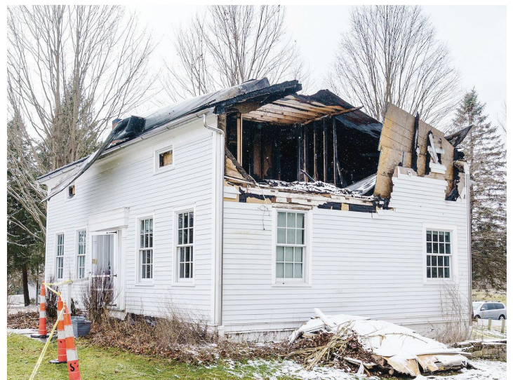
A third of the Heritage House roof is missing, along with a portion of wall on the eastern side.
